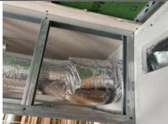
Photo 8.10. Example of thorough duct insulation and sealing.
