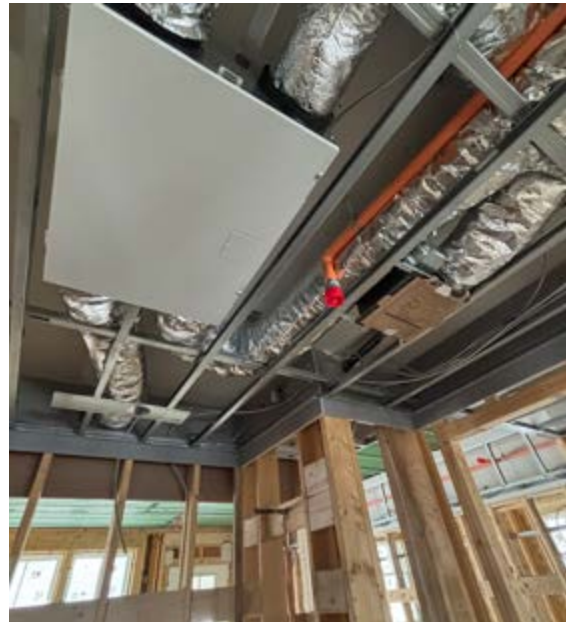
Photo 8.0. Substantial progress this period on rough plumbing, fire protection, mechanical and electrical.
