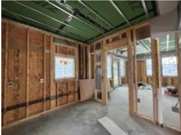
Photo 8.13. Some rough MEP progress in the common kitchen, common room and office.
