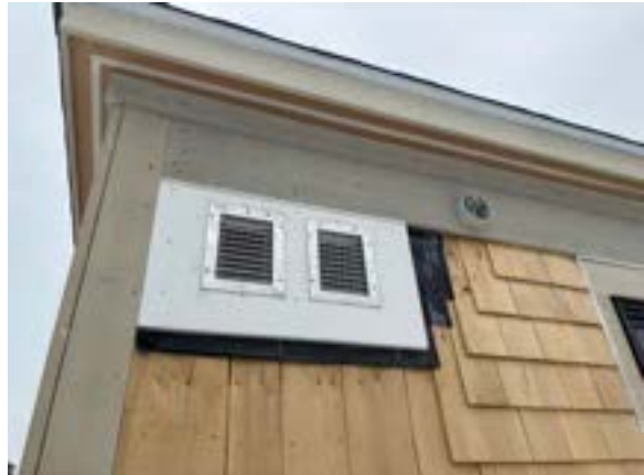
Photo 8.2. Substantial progress has been made on MEP penetrations, sealing and exterior trim.
