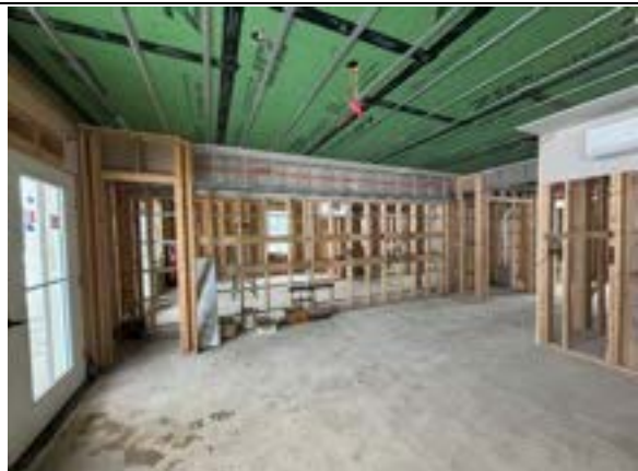
Photo 8.6. Typical east wing unit interior completion level. View from the living area towards the kitchen. Progress on all rough MEP trades.
