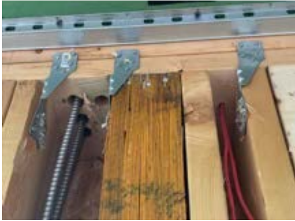
Photo 8.7. Holes have been drilled for electrical wiring. Careful attention to air sealing will be needed prior to covering.
