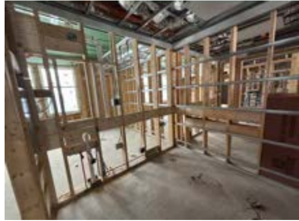
Photo 8.8. Typical east wing unit bathroom completion level. Progress on all rough MEP trades.
