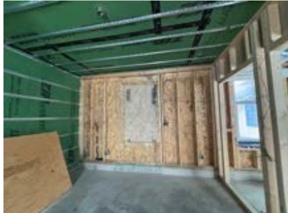
Photo 8.14. The wall and foundation of the office have been modified for the change from a window to a door.
