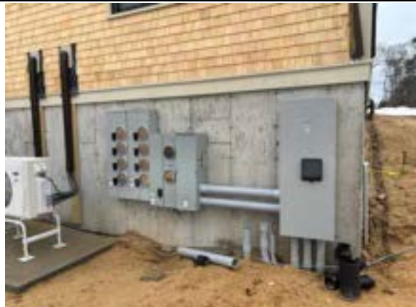
Photo 8.4. Electric meter work has started, addressing an issue that had previously been a bottleneck preventing subsequent work.
