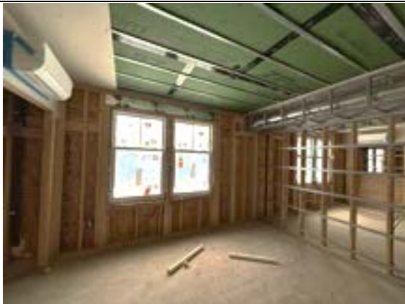
Photo 8.9. Typical east wing unit bedroom completion level. Progress on all rough MEP trades.
