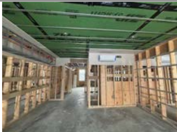
Photo 8.16. Typical north wing unit interior completion level. View from the living area towards the bathroom and bedroom with the kitchen to the left. Progress on all rough MEP trades, less than in the east wing.
