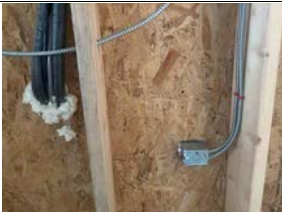
Photo 8.15. Some air sealing work at wall penetrations. Spray foam used at the refrigerant lines to the left, and nothing yet at the electrical box to the right.
