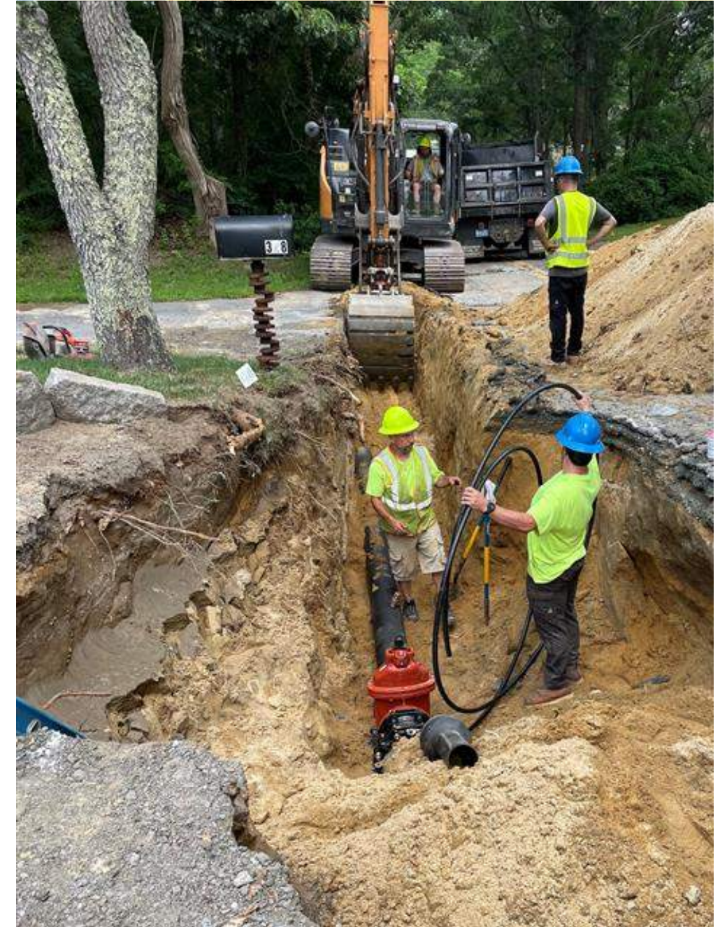
Example image showing typical placement of ductile iron water main in a roadway trench
